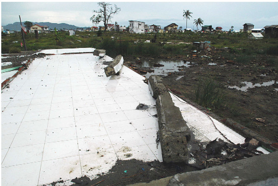
Fig. 5. Fallen columns in the Banda Aceh coastal plain indicating run-up tsunami direction.
