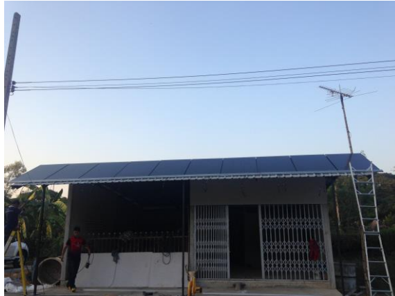
Figure 3 System of Roof Photovoltaic Array
