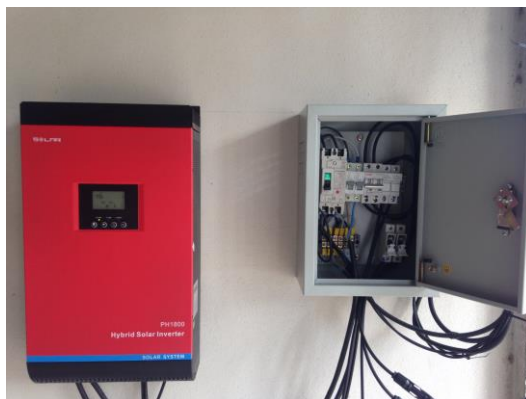
Figure 8 Inverter control system
